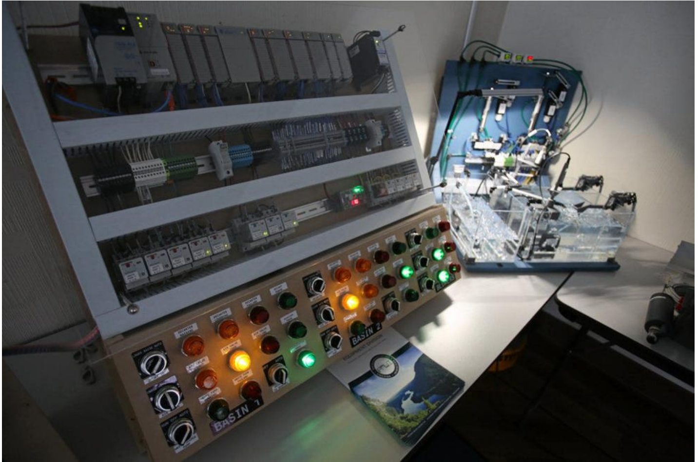
JAKE DANNA STEVENS / STAFF PHOTOGRAPHER The new control panel created by Pleasant Mount Welding Inc. in Carbondale will replace the larger control panel with multi-colored switches on the left.
